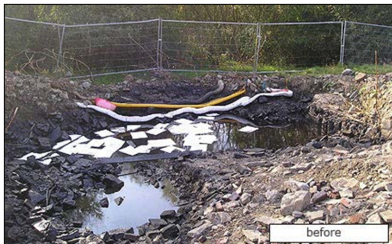
Waste oil contamination before remediation
